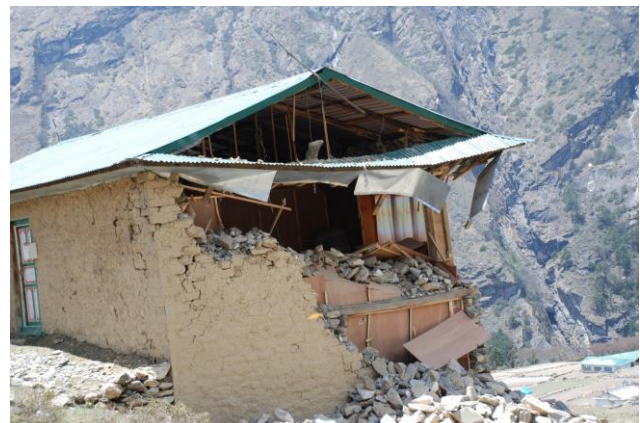
Fig. 6 Collapsed Community Center.
